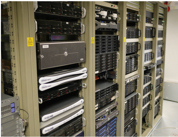
Visual Data DPP data center
